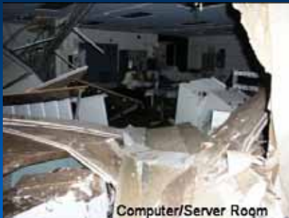
Flood Damage, University of Hawaii, October, 2004
